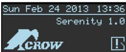
ZONE Tamper alarm
